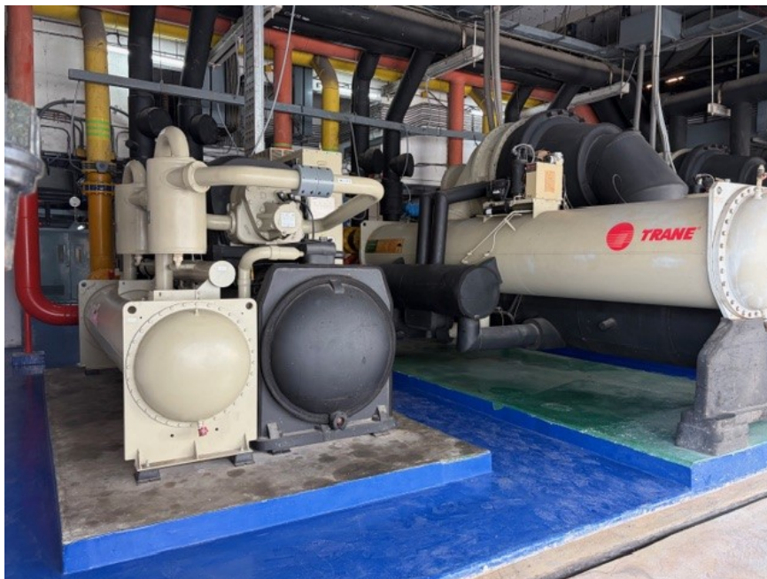
Chiller Plant System at JW Marriott Hotel
